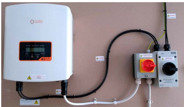
Figure 16: Installed inverter with electrical isolators
