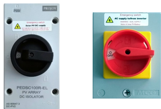
Figure 13. DC and AC isolators
